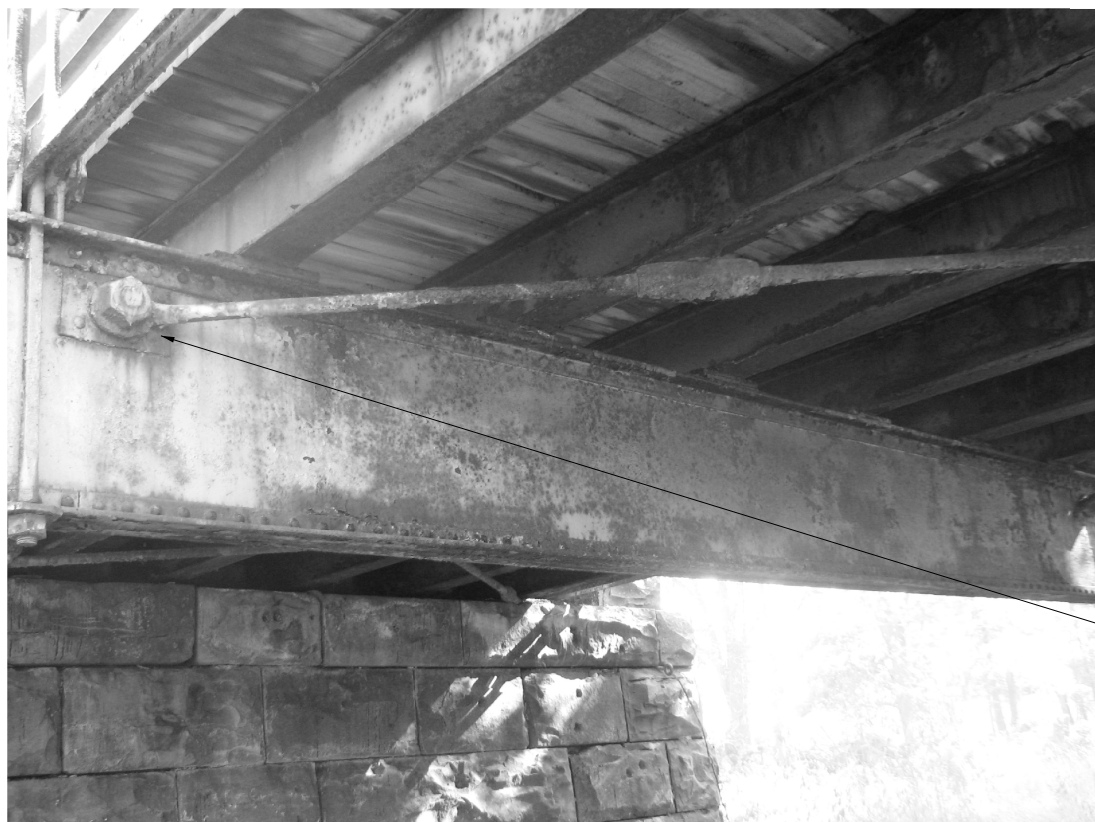
TYPICAL LOWER LATERAL BRACE TO FLOOR BEAM CONNECTION/ SAVE AND REFURBISH FLOOR BEAM AND LOWER LATERAL BRACING/ (REPLACE BOLTS, NUTS, AND REINFORCEMENT PLATES AT LOWER LATERAL CONNECTION POINTS. USE EXISTING BOLT, NUT, AND WASHER SIZES AS PROTOTYPE FOR NEW HARDWARE.) *
