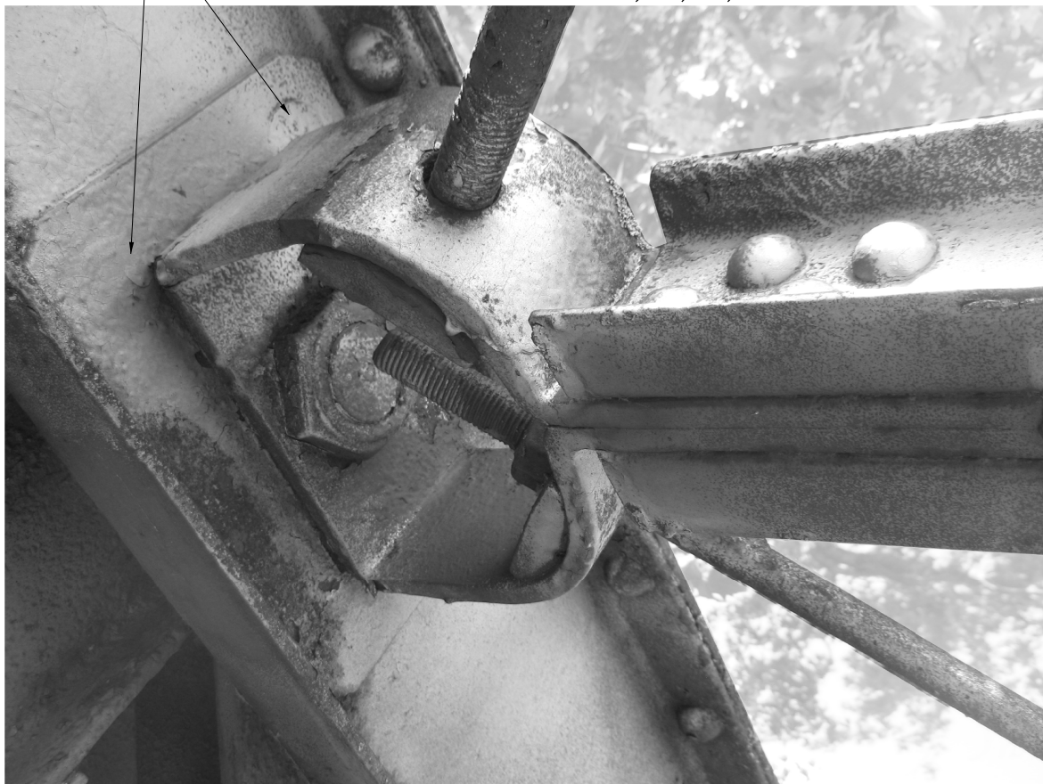
TYPICAL TOP STRUT TO TOP CHORD CONNECTION SAVE AND REFURBISH TOP CHORDS, TOP STRUTS, TOP LATERAL BRACES, AND CONNECTIONS. SEE NOTE PAGE 19/52 **
