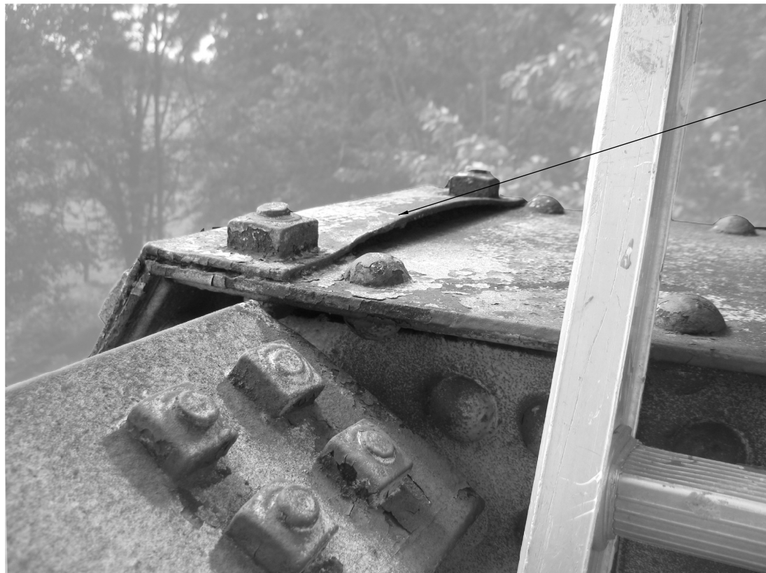
TYPICAL COVER PLATE AT END POST TO TOP CHORD CONNECTION ALL COVER PLATES SHALL BE REPLACED.
