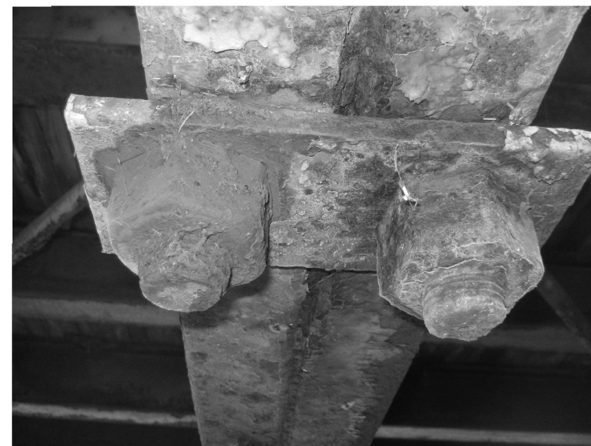
TYPICAL FLOOR BEAM TO TRUSS HANGER BOLT & PLATE REPLACE ALL HANGER BOLTS, NUTS, AND PLATES. SEE SHEET 40/52 FOR HANGER BOLT & PLATE DETAILS.
